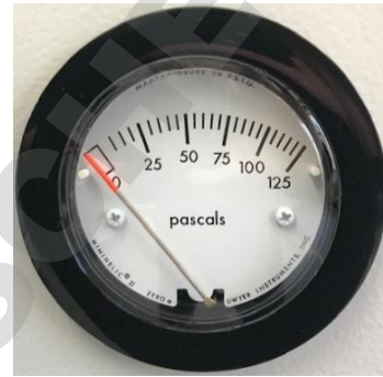
Figure 23: analog pressure display (manometer) for compressed air sweeping on the chamber front
