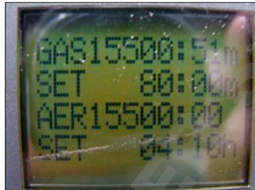
16. The timer on control panel starts:
