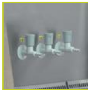
Media taps mounted on rear wall
