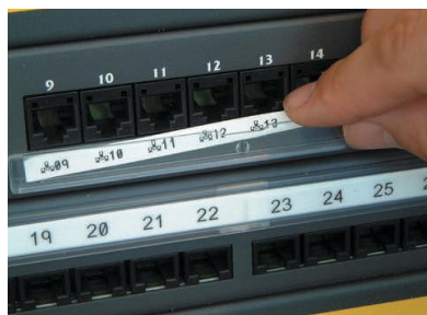
Punch block & patch panel labels
