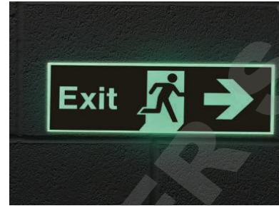
Exit & directional signs
