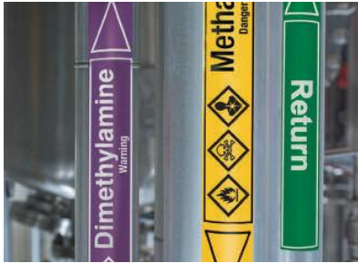
Pipe & valve marking
