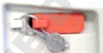
Locked with Wire Seal
